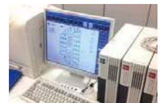
intelligent Manager is installed in the building's control room. Maintenance personnel have welcomed the system's straightforward setup and operation.
